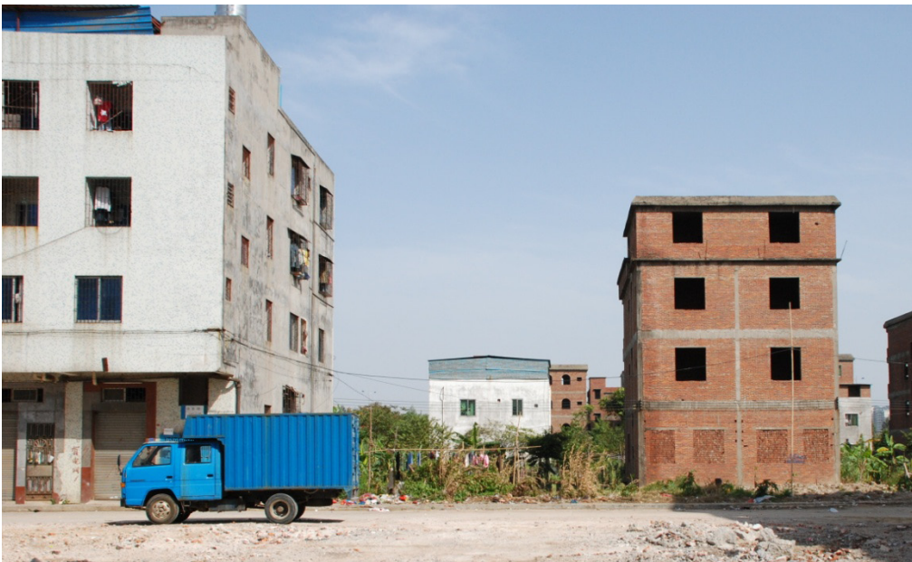
FIGURE 1: Jian Sha Zhou in 2008, half-completed buildings on the Danwei site. Image credit: Joshua Bolchover
